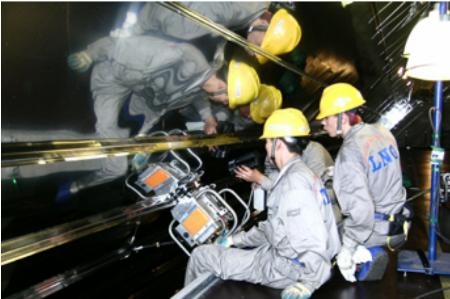
MASTERING THE TECHNOLOGY: Staff members from the China State Shipbuilding Corp. piece together an LNG ship
