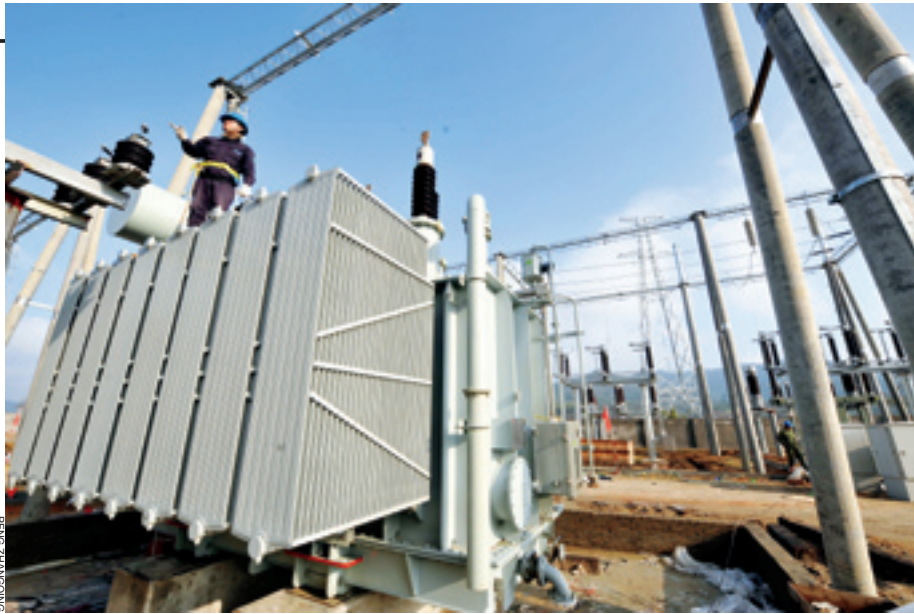
CONTROLLING FROM AFAR A worker conducts a final check on December 19 before the first 100-kw unmanned transformer substation in Shunchang County, Fujian Province, is put into use
