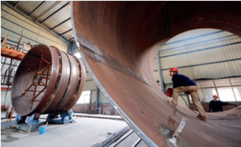
SPEEDING UP CONSTRUCTION Staff members work on steel penstocks at the Hongping Pumped-Storage Power Station in Jiangxi Province on December 5
