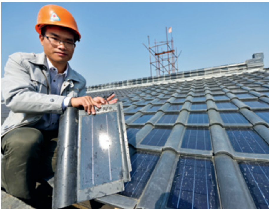
POWER ON A worker installs photovoltaic ceramic roofing in a village in east China's Zhejiang Province on November 14. The generated power will be used for household electricity consumption
