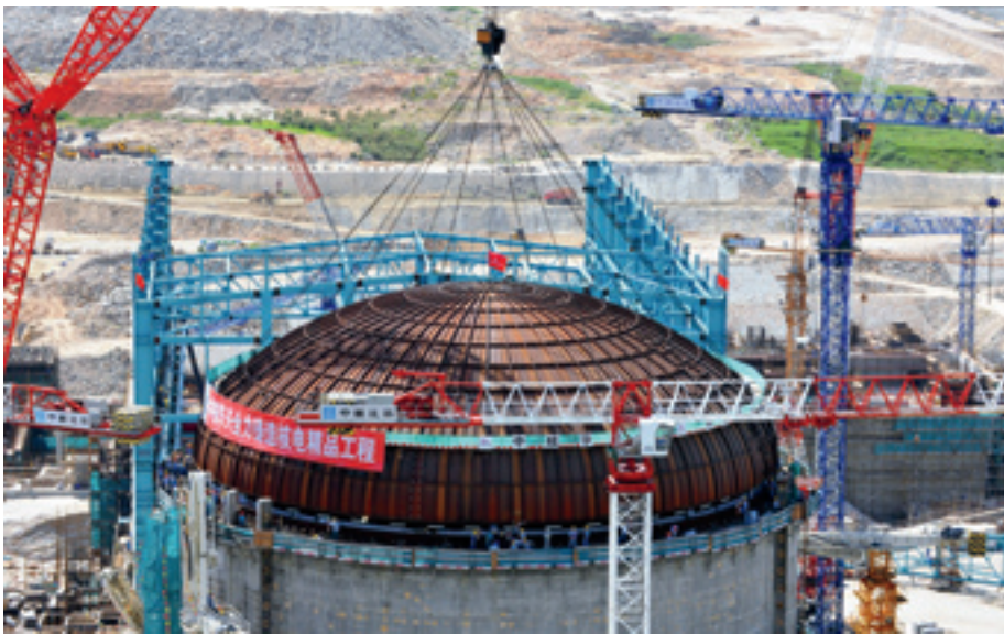
SUCCESSFUL CAPPING A dome is fitted onto the second reactor building of the Taishan Nuclear Power Station on September 12. Located in Jiangmen, Guangdong Province, the station has two European pressurized reactors, with a total installed capacity of 3.5 million kw
