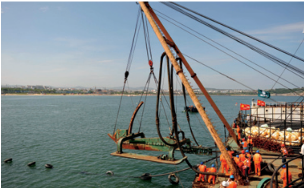
UNDERSEA CABLE A 3,000-ton ship lays undersea cables at Penglai Port of Shandong Peninsula on September 2. The cable will carry electricity to the Changdao Islands in the Bohai Sea
