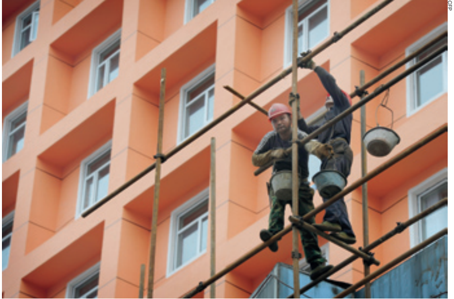
HIGH ABOVE GROUND: Construction workers work on scaffolding at a housing project in Nanjing, Jiangsu Province, on June 30
