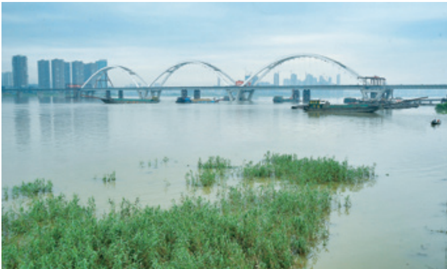
NEW BRIDGE Xiangjiang Bridge on Fuyuan Road of Changsha, central China's Hunan Province, finishes the main body construction on July 18 and will be put into use in October
