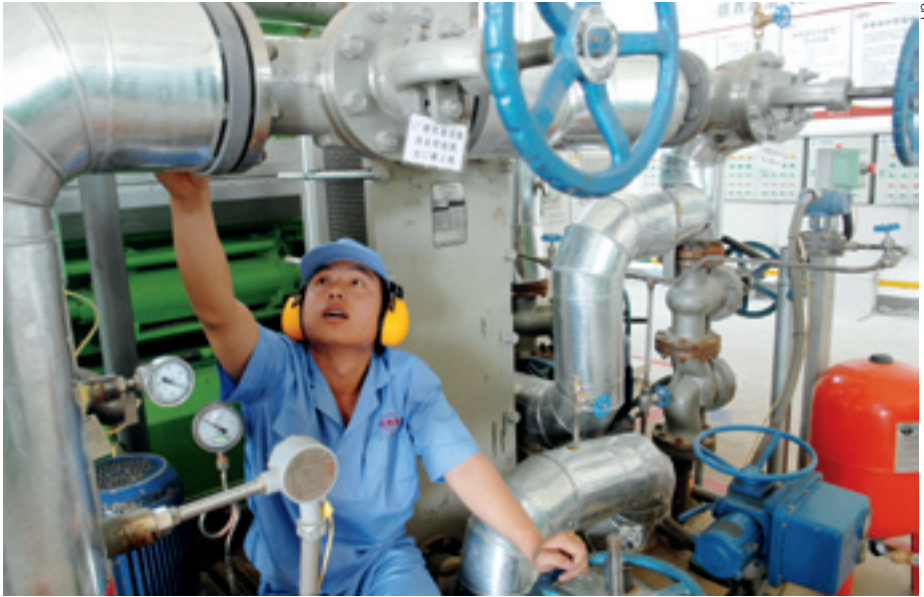
POWER ON: A worker monitors generating sets in a DQY biogas power plant in Yanqing County, Beijing on May 19, 2009
