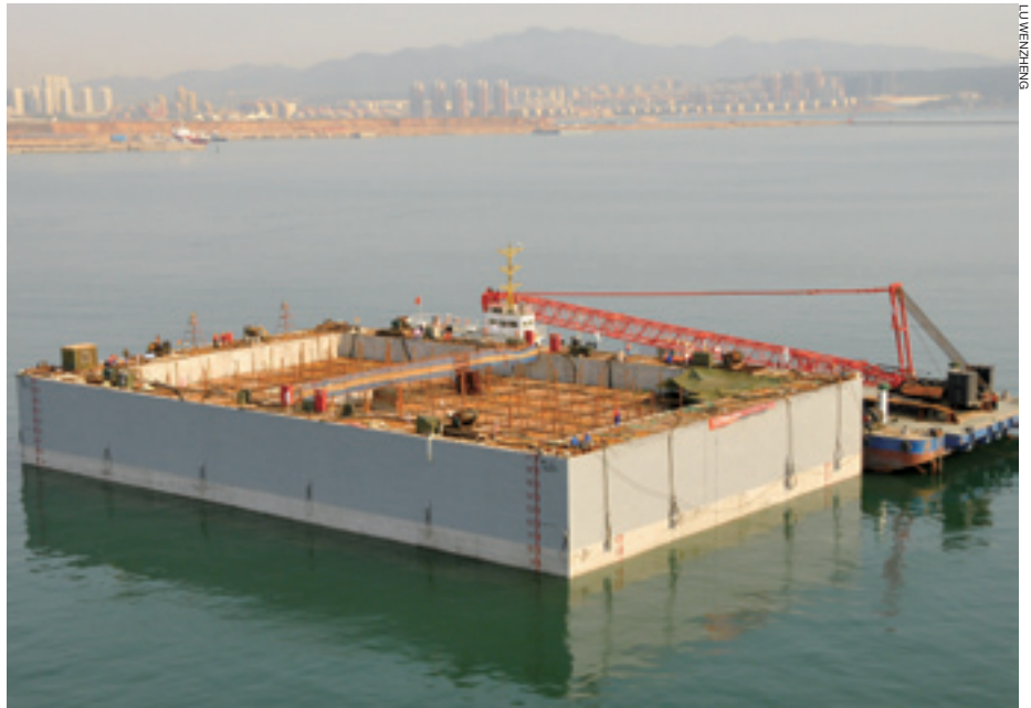
FUTURE CONNECTION A bridge pier weighing 26,000 tons is fixed in place to the Xinghai Bay Cross-Sea Bridge in Dalian, Liaoning Province, on May 16. The bridge with a length of 5.3 km connects the urban district of Dalian to its Hi-tech Industrial Zone and will open for traffic in 2013
