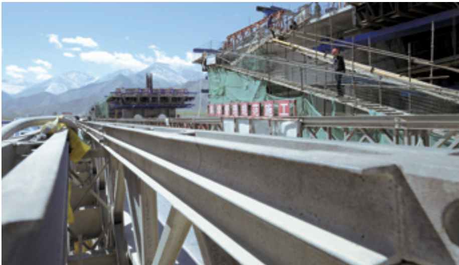
NEW CONNECTION The bridge across Lhasa River in Lhasa, capital of west China's Tibet Autonomous Region, is under construction. The 1.28-km bridge, called the No.1 bridge in Lhasa, will be finished in October
