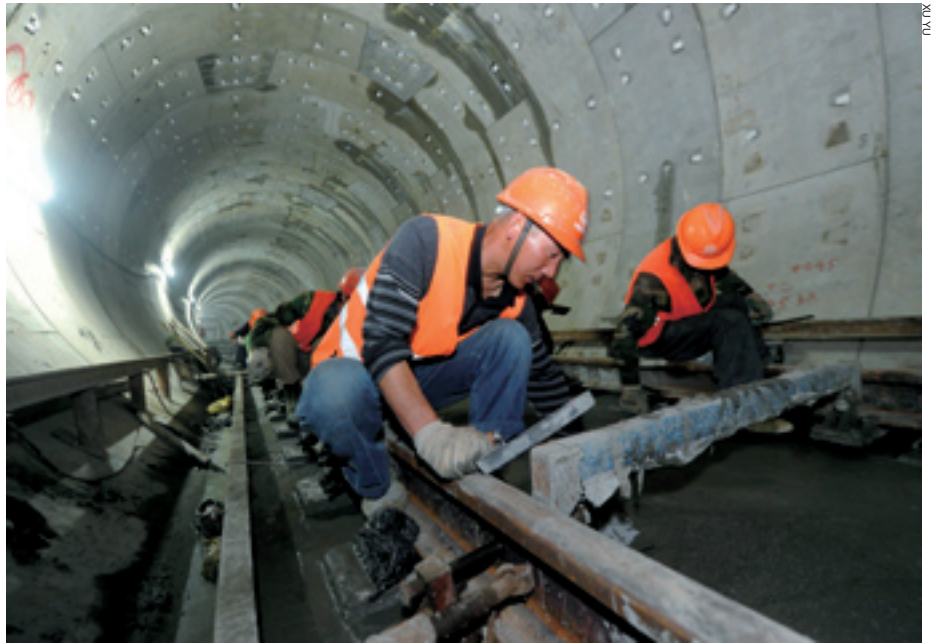
BRIDGING HANGZHOU Engineers work on the project of Subway Line 1 in Hangzhou, capital of east China's Zhejiang Province, which is scheduled to begin trial operation in June 2012
